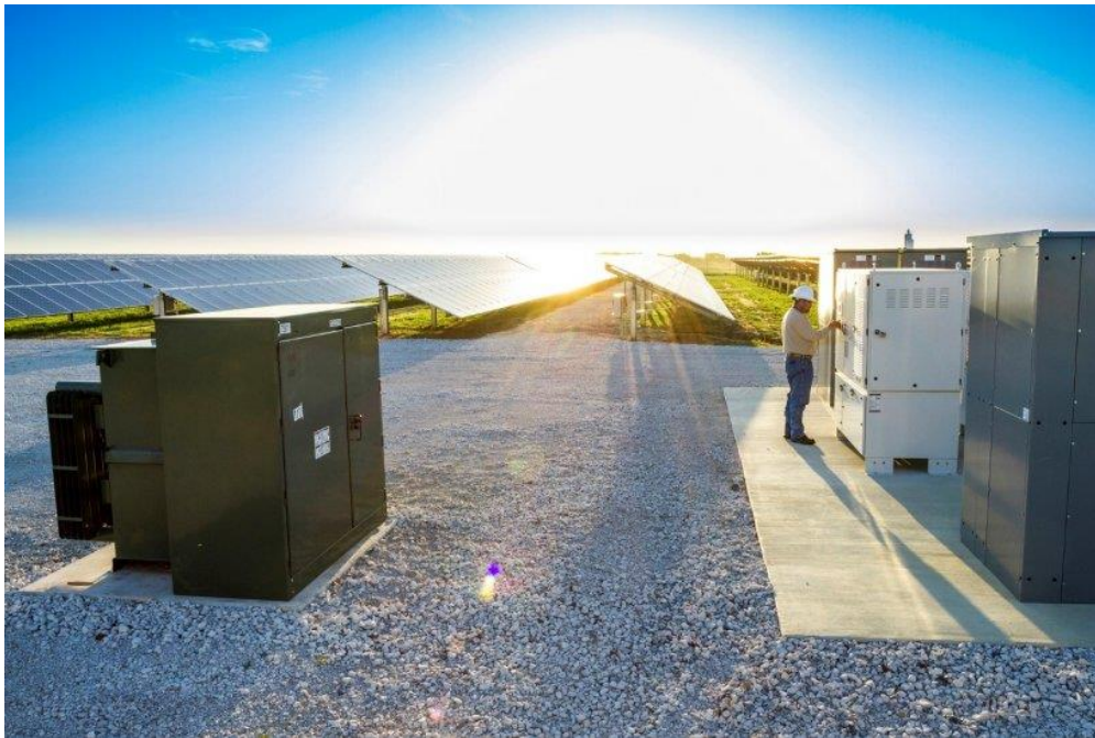
A worker checks an inverter at the 2MW CoServ Solar Station in Krugerville, Texas. Photo by Ken Oltmann/CoServ.
